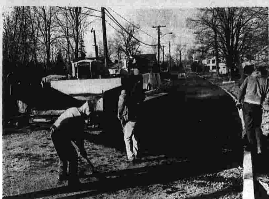
Workers from Della Construction Co. spread pavement on Adams St. Thursday. A stretch of the road from Bigelow Brook to Hilliard St. was paved, completing paving that will be finished in the spring. (Herald photo by Dunn)
